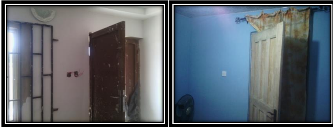
Figure 4: Poorly executed electrical installations/fittings: the doors open to cover the main-switches.
