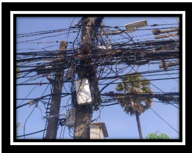
Figure 6: A functional but aesthetically poor and hazardous electrical installation. Source: Arrive Alive (2018).
