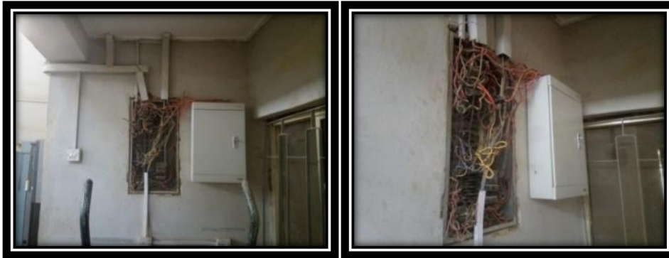
Figure 2A and B: A poorly executed electrical installation: untidy and aesthetically assaulting. It is a common feature in many Nigerian buildings or structures.
