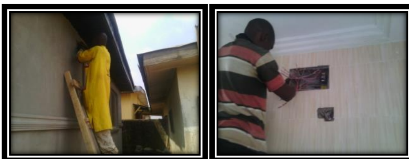
Figures 3a and b: Non-formally educated electricians at work in the study area.
